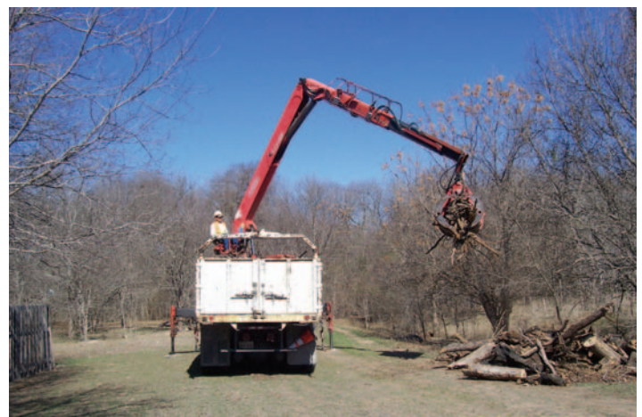
City of Austin employee Frankie Andrada with Watershed Protection Department airlifts dead brush and logs from the Onion Creek greenbelt behind Wild Dunes Drive. Crews removed the brush after geotechnical investigations in this area were done for preliminary engineering of the wastewater interceptors.
